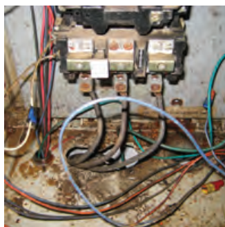
Corrosion leads to premature component failure
