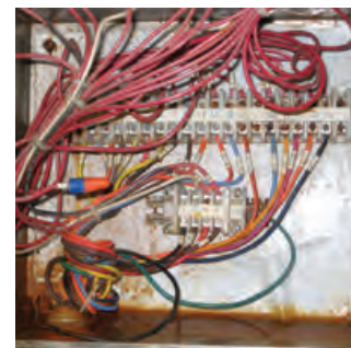
Water accumulation in electrical cabinet
