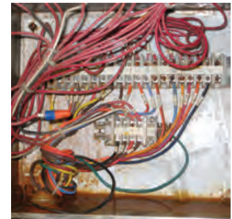
Water accumulation in electrical cabinet
