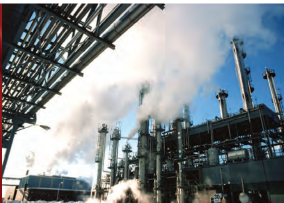
Instrumentation and Automated Pneumatic Controls
